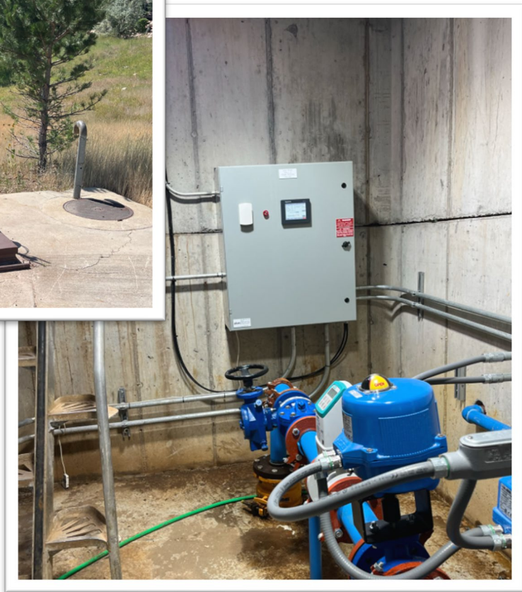
New Telemetry, SCADA, and Electrical at Sun Peak Well 2
