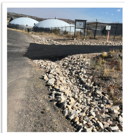
Paving and drainage improvements at Silver Creek. Relocated material storage shown in upper photo.
