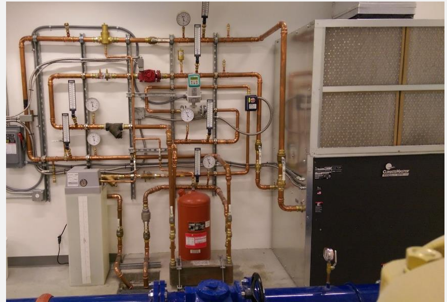
Geothermal cooling system
