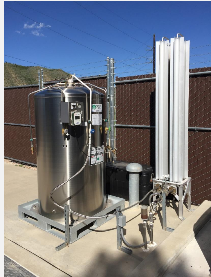
Liquid nitrogen system
