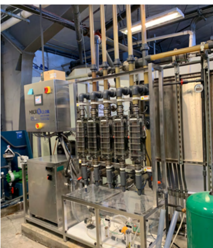
Chlorine Generation System
