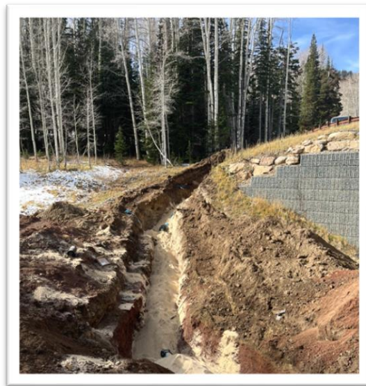
New Water Line being Installed at the Last Chance Subdivision (Upper Colony)
