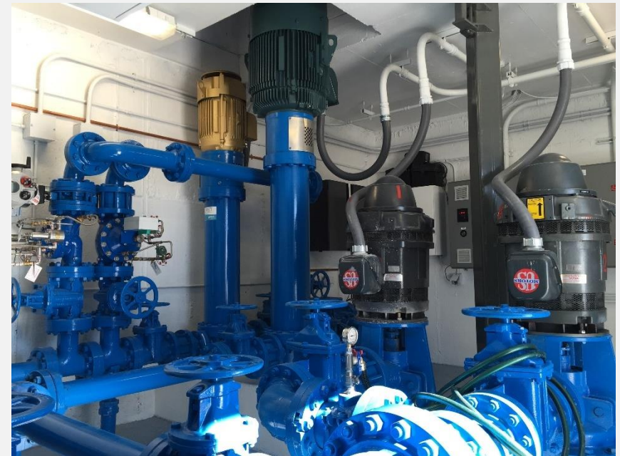
Blackhawk Pump Station Upgrades
