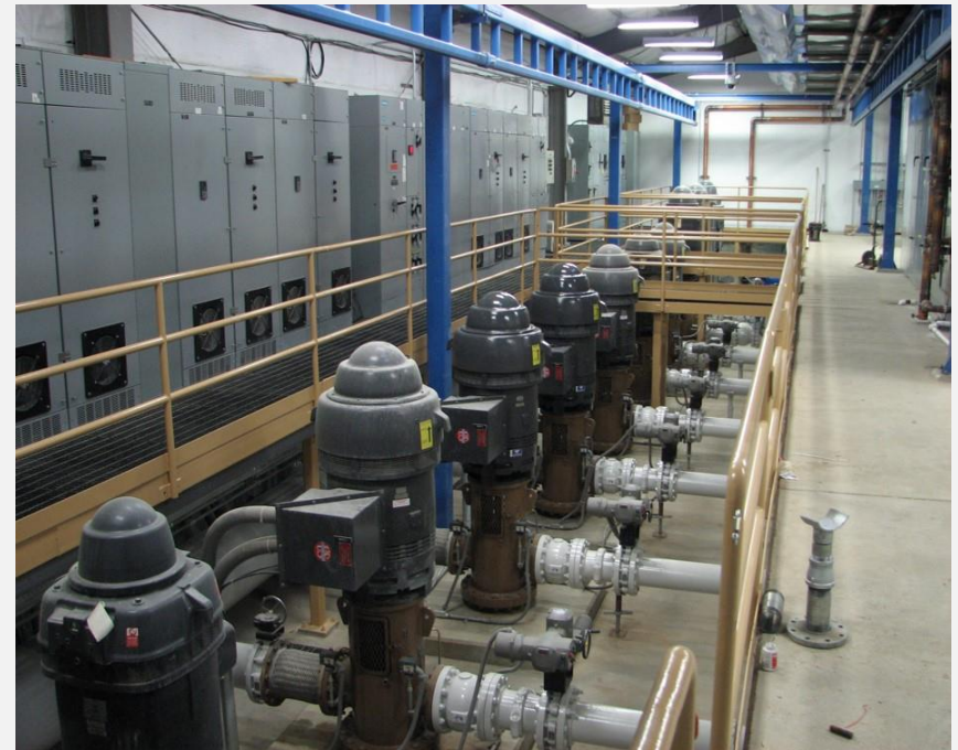
Lost Canyon Booster Station
